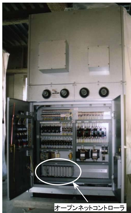
図 16 空調機本体と制御盤 Fig. 16 Air Conditioning Equipment and Control Panel
