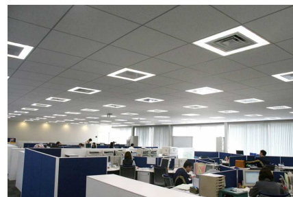
図 2 2 階オフィスの LED 照明の様子 Fig.2 Photograph of the office with LED lighting
