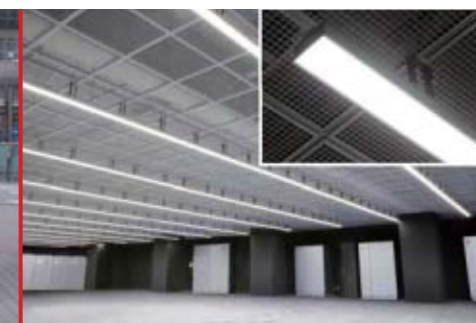
January: TIS Inc. Delivered LED base lighting to "GDC Gotenyama", a next-generation data center
