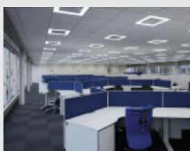
Example of LED lighting control system in the office
